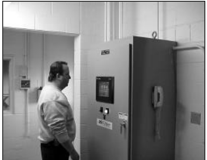
Utilities Operations Supervisor Dave Pearson is shown above checking the operational set points on programmable logic controls at Well #10.
