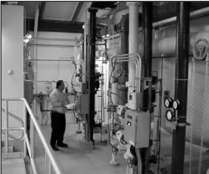
Village of Lake Zurich Utilities Operations Supervisor Dave Pearson records water flow rates at Well #10.
