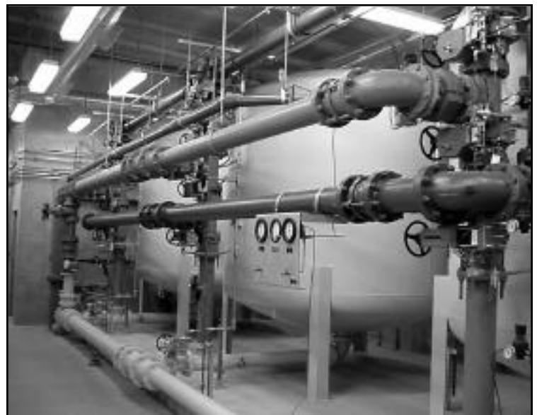
ION Exchange vessels and face piping at Well 8.
